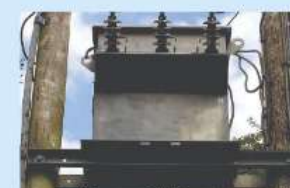
Separate Electric Transformer
